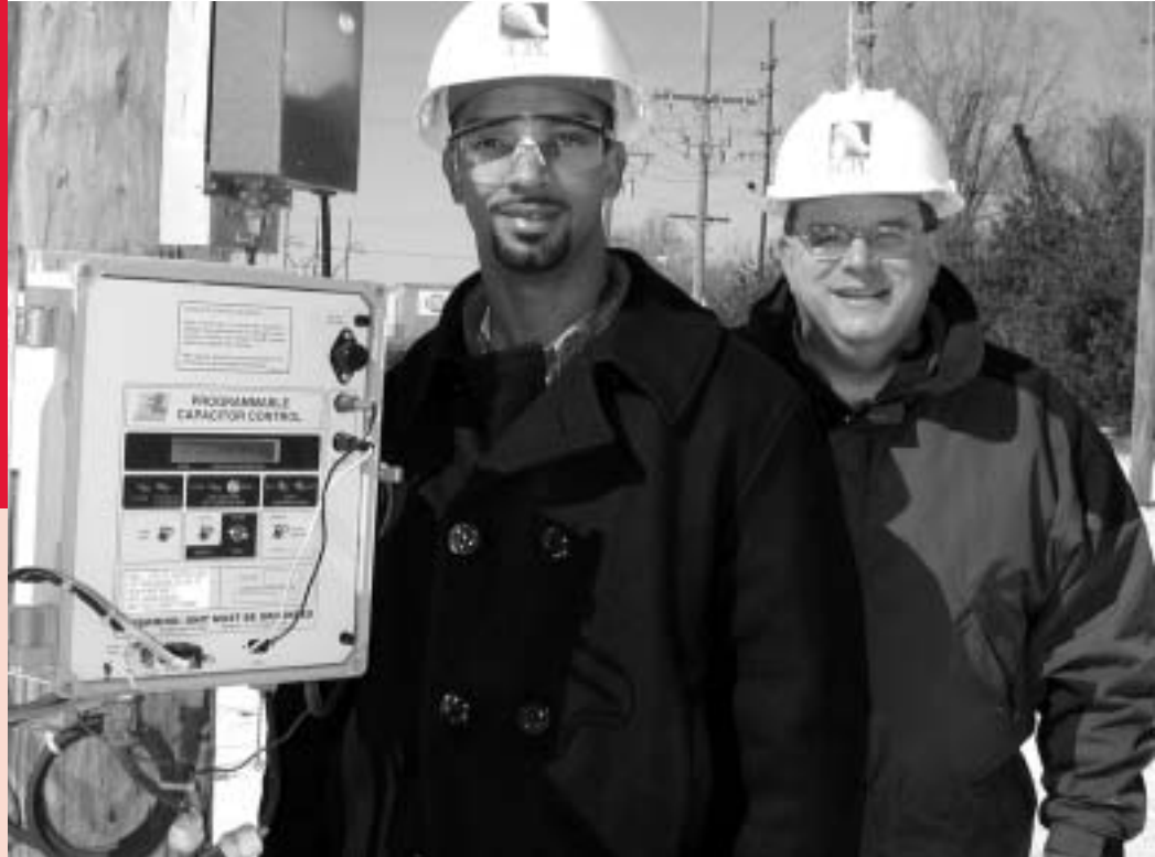
Philip Cosey III, left, and Carl Goeckeler, distribution automation engineers, led KCP&L's project team honored by Utility Automation & Engineering T&D Magazine . The two devices on the pole are integral components of the team's new award-winning concept.
