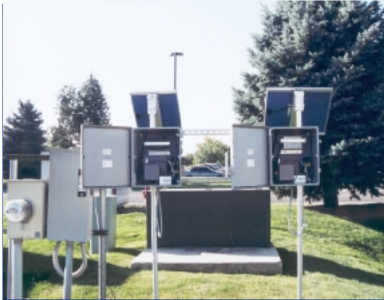
The Remote Wireless Control System
