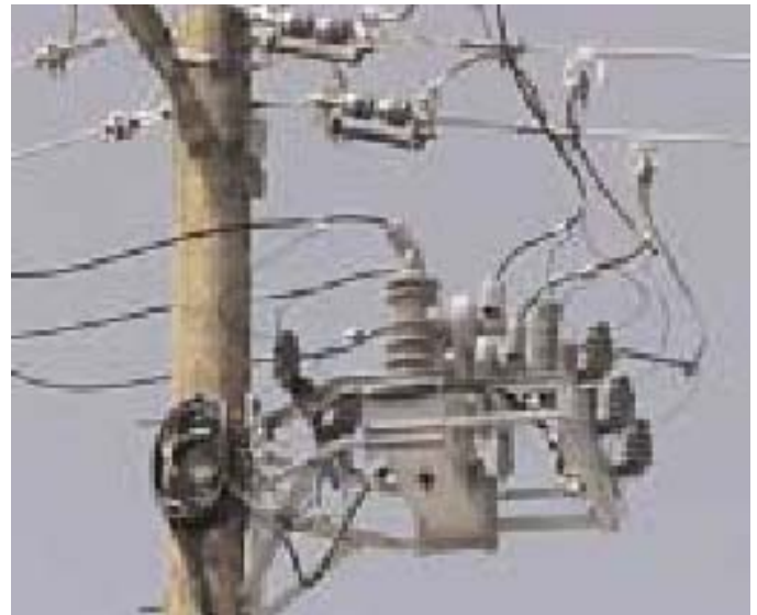
Cooper Recloser on overhead feeder
