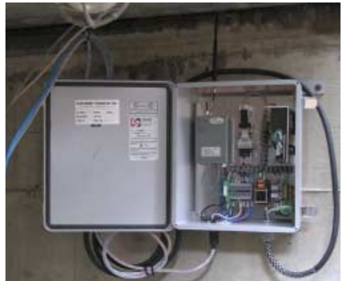
Typical Installation of Concentrator Box at the Top of a Network Vault.
