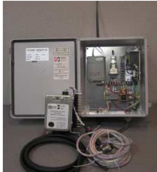
ETI Concentrator Box with Telemetric DNP-RTM, power supply and harnesses for connecting to ETI MNPR network protector relay (also shown).
